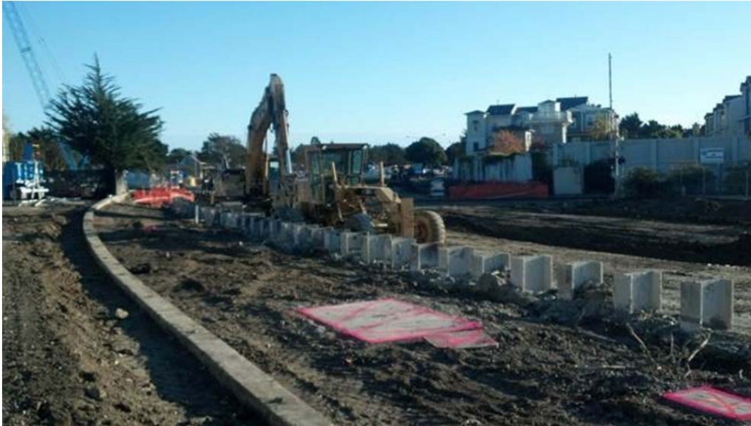
Photo of a section of completed DSM wall. The vertical steel I-beams extend below grade approximately 60 feet and are encased in a hardened concrete mixture.
